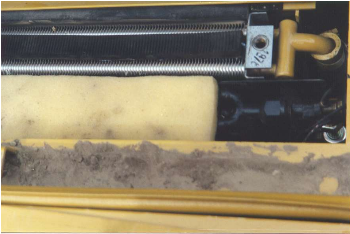
Top of evaporator assembly in heater box.
