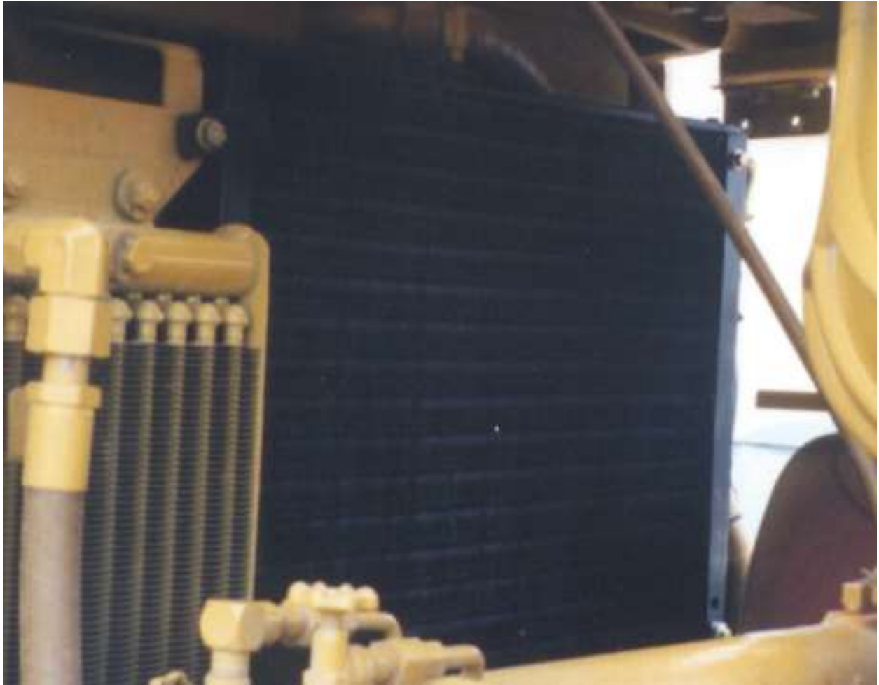
Left side of the condenser with hold down brackets in place.
